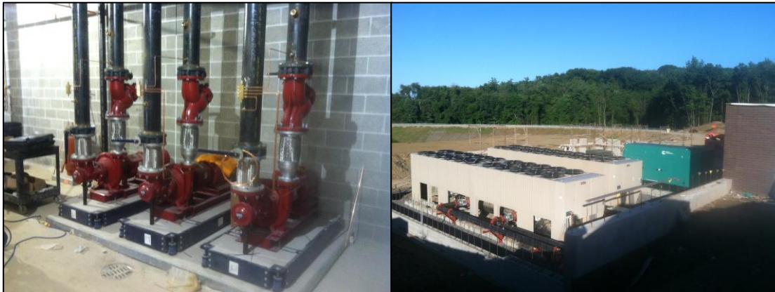
Figure 6: CHWPs & Chiller Yard (Mascaro Property)
