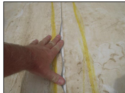
Figure 67: TPO Failure at CWNCHS (Florida Consulting Property)
