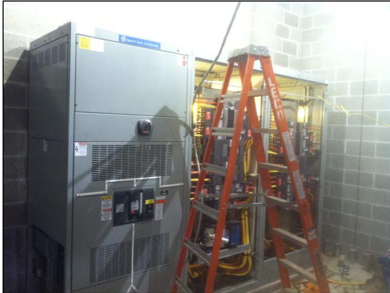
Figure 7: 3,000A Main Switchboard (Mascaro Property)
